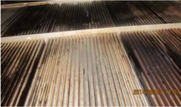
Figure 2. Severe fouling between tube bundles
