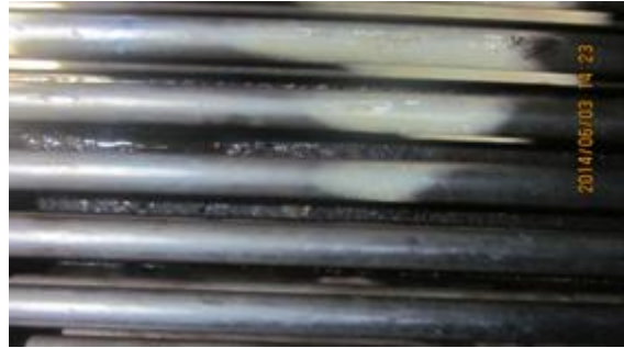
Figure 3. Severe fouling between tube bundles
