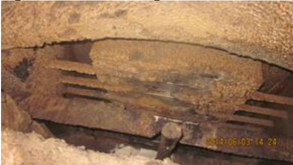
Figure 4. Thick dirt covering mist eliminator
