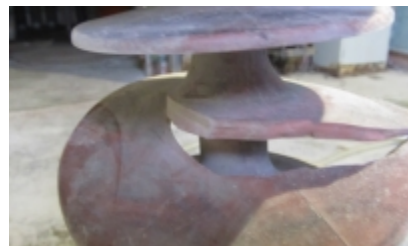
Fig.1 Damage and brittleness of insulator umbrella skirt
