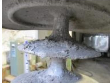
Fig.2 Insulator contamination situation
