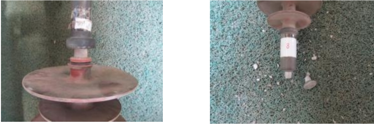
Fig.4 Mechanical disruption of insulators
