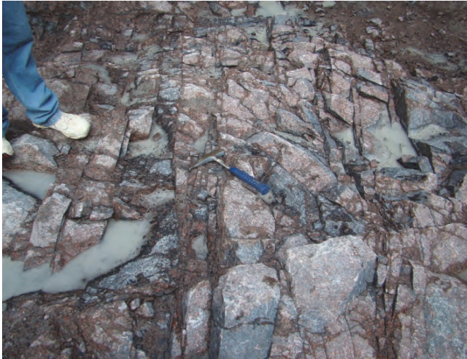
Fig. 5. Prominent joints at the foundation of Pump house
