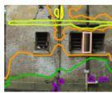
Fig. 10. Outlines of various defects.
