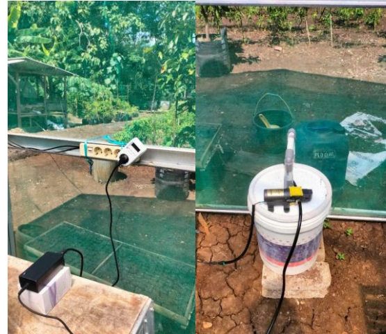
Figure 3 Timer and pump for the automatic watering system
