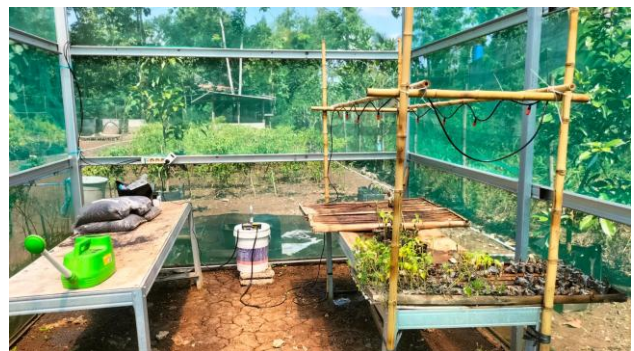
Figure 4 Automatic watering system for greenhouse .
