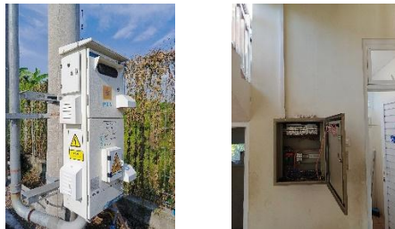
Fig. 6. KWH Meter Location Points and Share Panels
