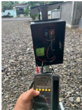
Fig. 8. Power Testing on Solar Panels. Source : Personal Documentation.
