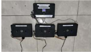
Fig. 10. Transmitter Node & Receiver Node
