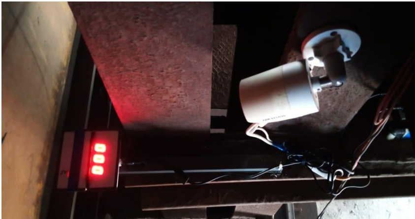
Fig. 4. Sensor counter installed near runway girder to count crane trips.
