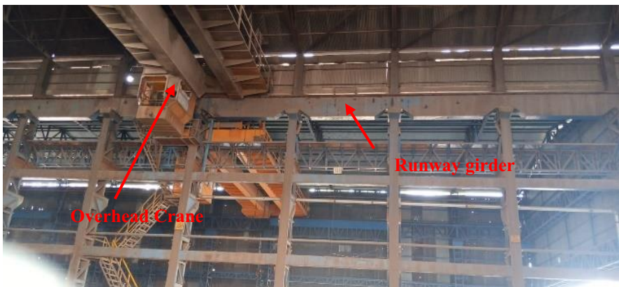
Fig. 2. Image of the Crane girder having overhead crane supported on columns bracket.
