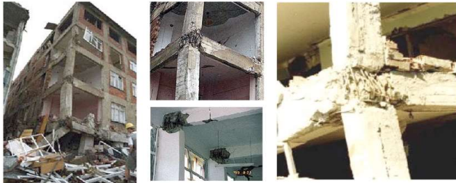
Figure 2. Collapse of structures due to failure of connections [4]
