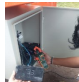
Figure 16. Measuring motor current, component voltage and motor speed
