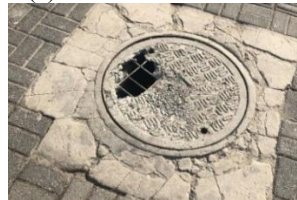
(d) Defects in the well cover
