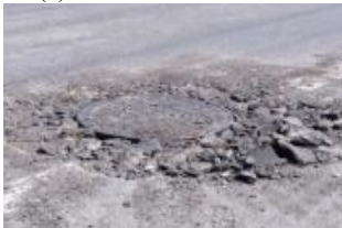
(c) Damage around the well
