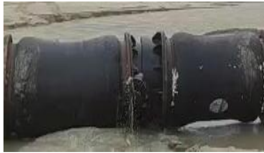
Fig. 9. Both ends of the socket pipe joint are rubber pipes
