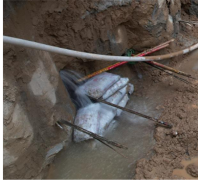
Fig. 3. Anchor Cable Hole Leakage
