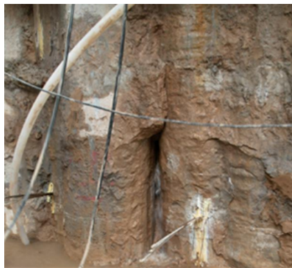
Fig. 2. Water seepage between interlocking piles
