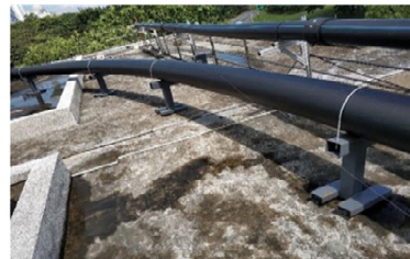
(b) Flexible monitoring pipeline
