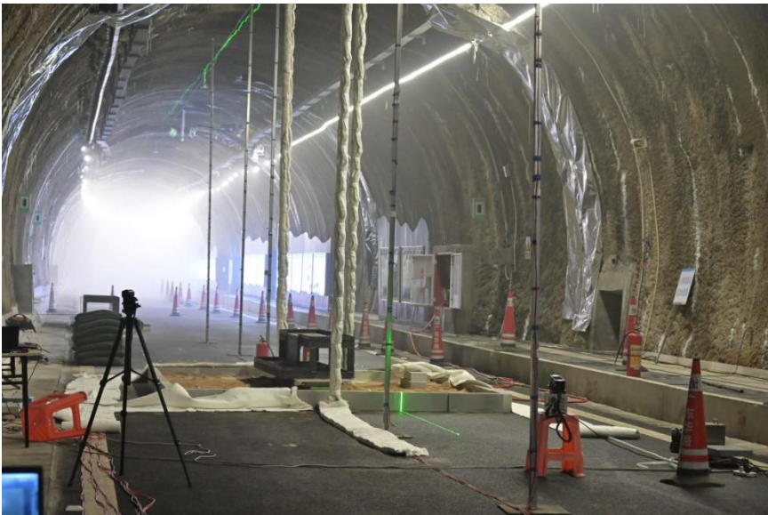
(b) After the "one-key linkage" control plan of tunnel electromechanical equipment is started (flue gas discharge tunnel)
