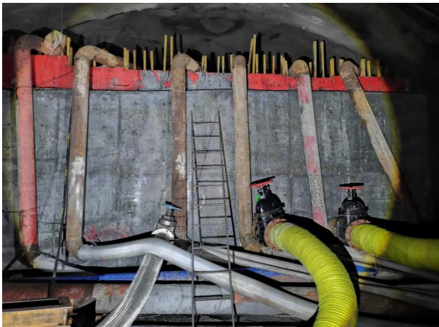
Fig. 4. Refuge Bay Water Storage Tank.
