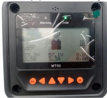
Figure 3. Monitoring the electrical energy produced
