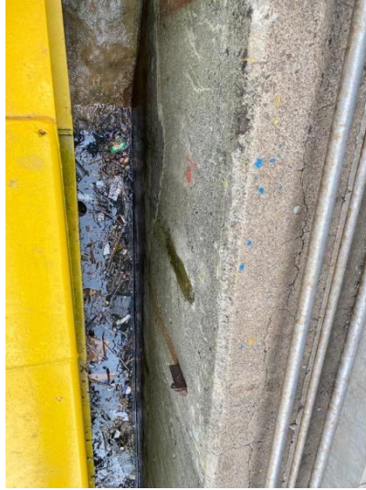
Fig. 2. Garbage piled up on the edge of the pontoon.
