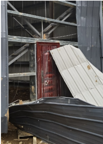
(a)The blast face is damaged
