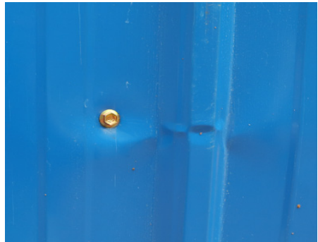
(b) Purlin contact damaged
