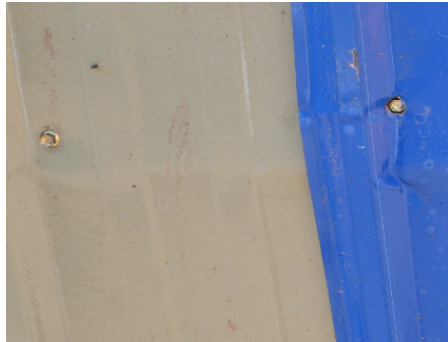
(b) Purlin contact damaged
