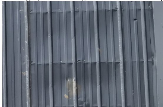
Fig. 6. The blasting surface is deformed
