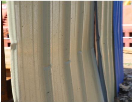
(a) The steel plate is damaged in the longitudinal span
