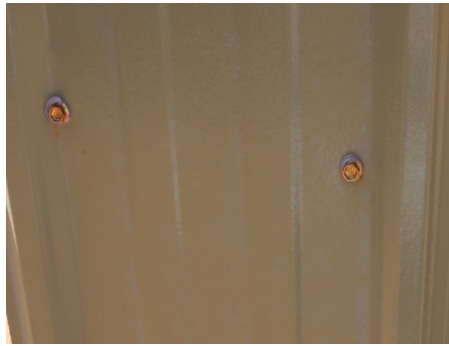
(b) Purlin contact damaged
