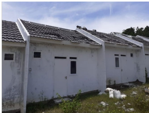
Fig. 1. Tile damage on a housing in Duta Pakis Residence, Indonesia.
