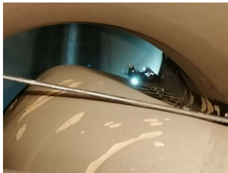
Fig. 2. Steel-lining bulge photos in 2020
