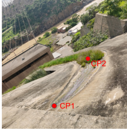
Fig. 5. Water leakage points on the outer concrete at the inclined pipe section of penstock
