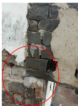
Fig. 12. The plastering layer on the outer wall of the stone-wood structure peels off
