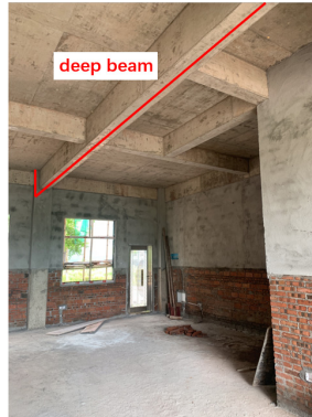
Fig. 21. A frame structure under construction replaces the bottom middle frame column with a deep beam
