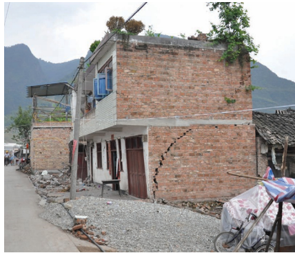
Fig. 18. A two-story cantilevered brick-concrete structure was damaged in Lushan earthquake.
