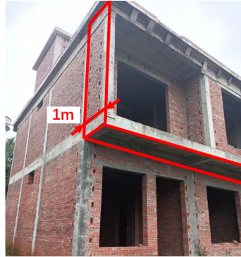
Fig. 17. A brick-concrete structure under construction in a township of Hainan Province has a cantilevered part on its second floor
