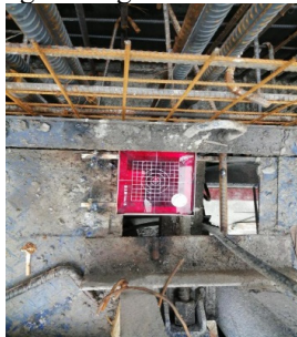
Fig. 3. Fast monitoring device of laser plumb bob.
