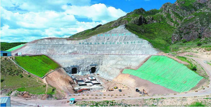
Fig. 8. Exit of the sand tunnel in the lower reservoir of a pumped storage power station (This image comes from the Internet)
