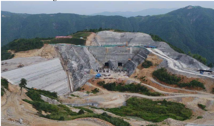
Fig. 10. Construction of the upper water inlet / outlet outlet of a pumped storage power station (This image comes from the Internet)
