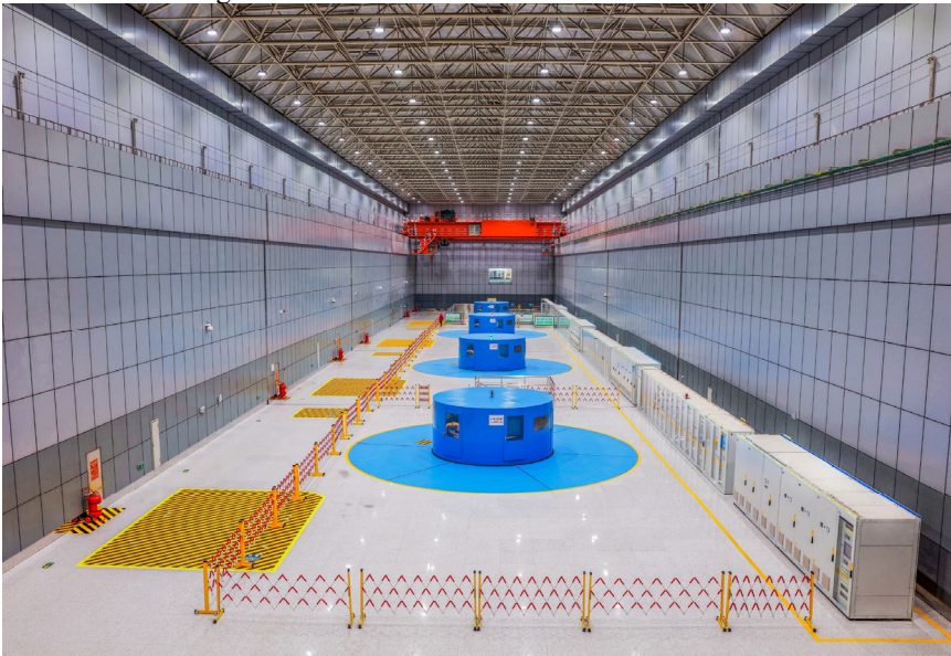
Fig. 7. The underground workshop of a pumped storage power station (This image comes from the Internet)
