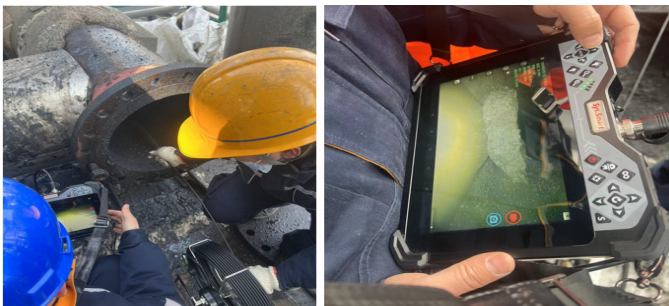
Fig. 1. The detection robot in the pipeline of coking unit finds the coke blocking position
