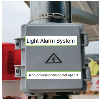
Fig. 5. Sound and light alarm system and safety indicator
