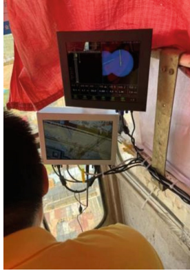
Fig. 3. Tower crane hook visualization system
