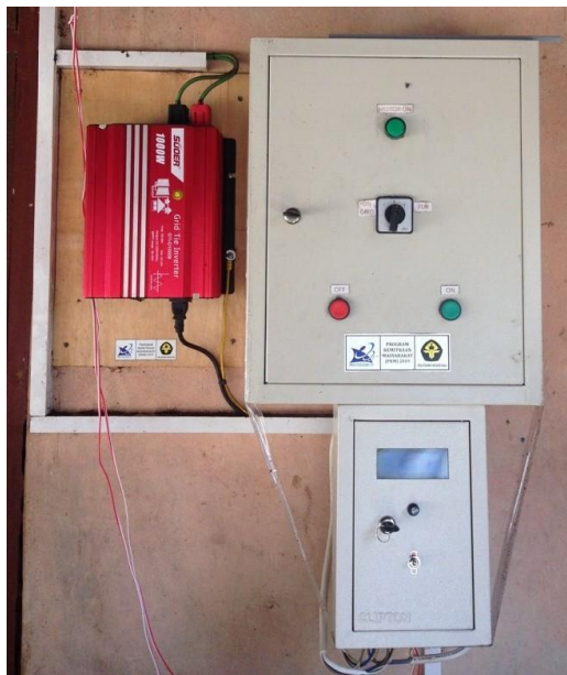
Fig. 8. Monitoring system panel under the solar power system panel.
